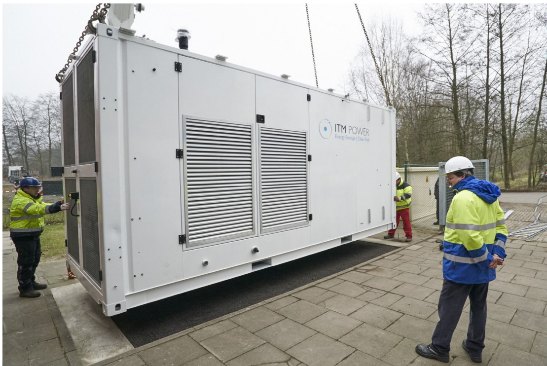
ITM Power-to-Gas PEM electrolyser system
