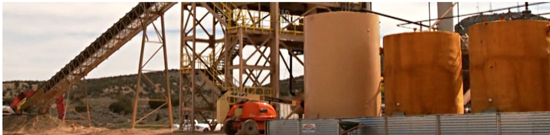
Petroteq's oil sands processing facility. Source: Company
