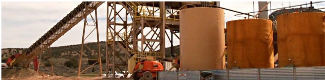
Petroteq's oil sands processing facility. Source: Company
