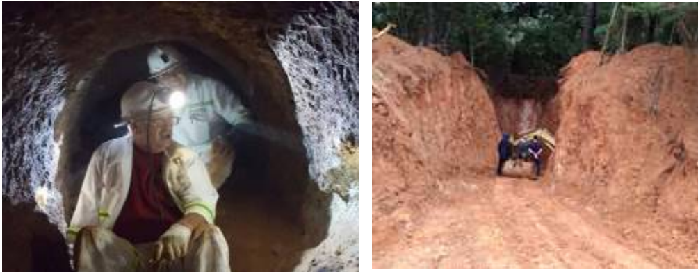
Work begins at Gubong (left) and track to access an inclined shaft (right). Source: Company & CPR January 2018.
